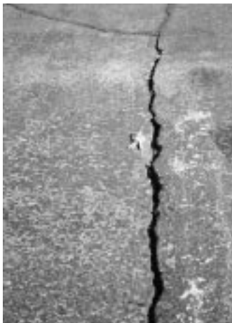
▲ Open crack – 1/2" or more in width.
