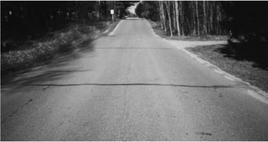
▼ Widely spaced, well-sealed cracks.
